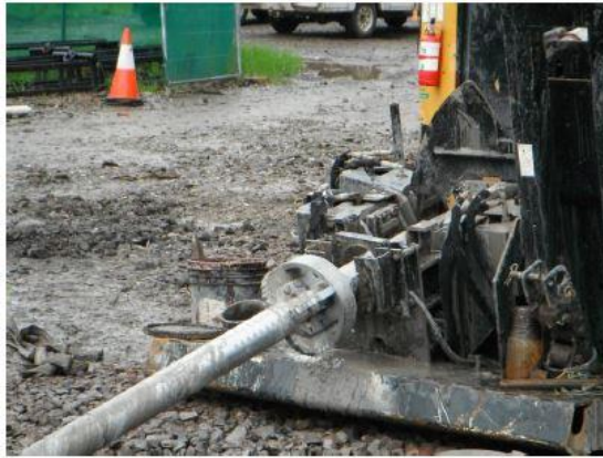
The tungsten carbide cutters were replaced with PDC ones on site in less than an hour
